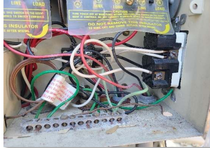
Photo of control panel interior
