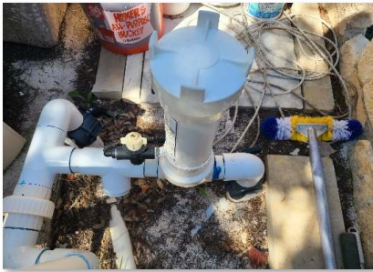
Photo of water sanitization device (OK)
