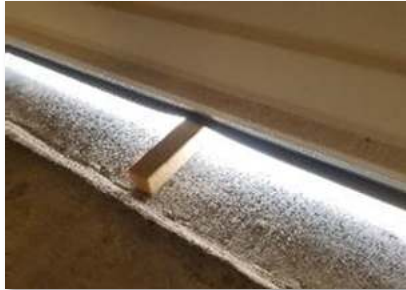
Item C (failed test)
