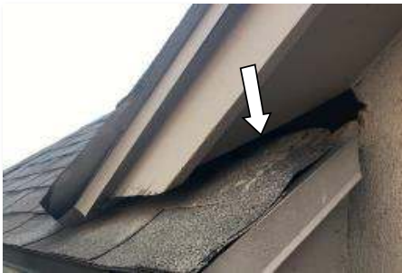
Item A (sample of rodent entry point)
