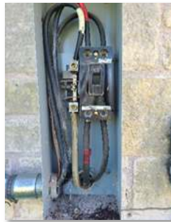
Interior of service panel
