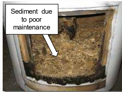
Item A (sediment buildup)
