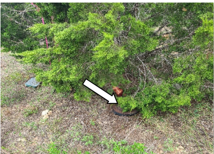
Location of water shutoff / meter
