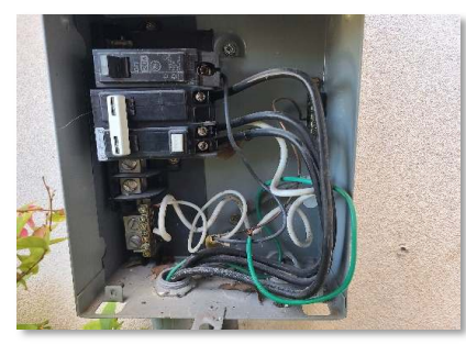
Interior of subpanel by rear patio
