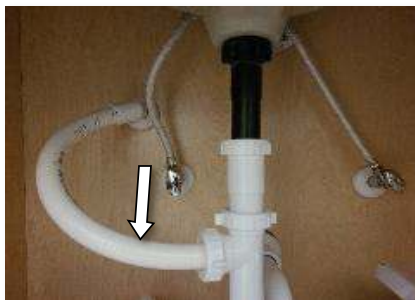
Item B (sample of condensate at sink)
