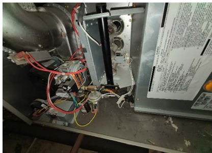
Interior of HVAC unit (OK)
