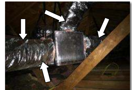
Item F5 (poor distribution box)
